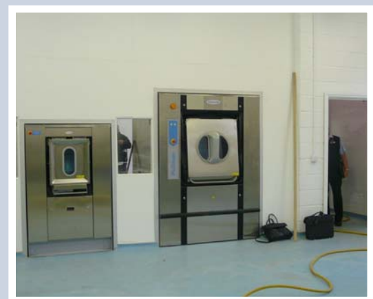
The body of the machines sit in the dirty side. On the clean side they are flush to the barrier wall (as above).
