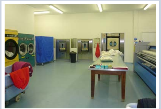
The clean side. Laundry to be tumble dried goes along one side of the room and flatwork to be ironed flows along the other side.
